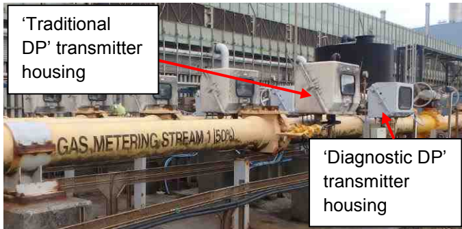
Figure 22 - AGI gas metering skid with instrument enclosures
