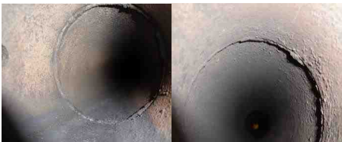
Figure 17 - Upstream (left) and downstream (right) meter run
